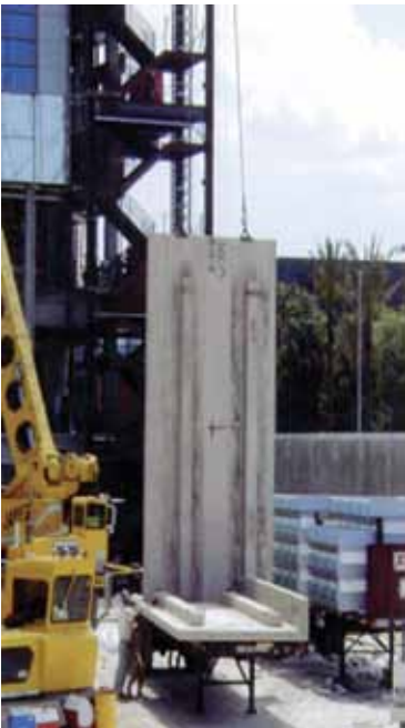
Figure 8 The 6 in. thick x 22 ft. tall panels were reinforced with ribs spaced 6 ft. apart.
